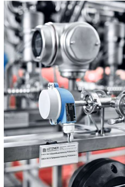
Measurement technology in the test bench: in front fast responding temperature sensors of type iTHERM TM411 with QuickSens technology, in the background mass flow meters of type Promass E 300 and pressure transmitters of type Cerabar M PMP55.
