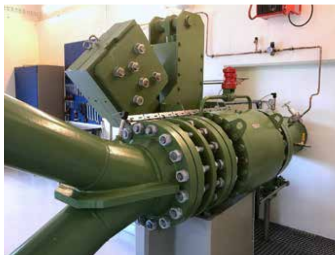
Ball valve at the Norwegian Liarelva hydroelectric power plant
